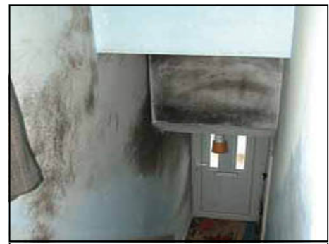
Extensive mould growth to stairwell
