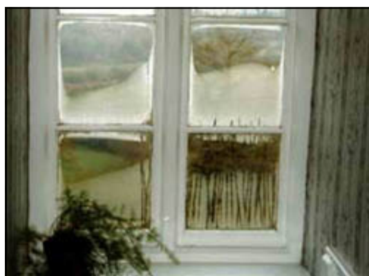
Typical condensation on a window
